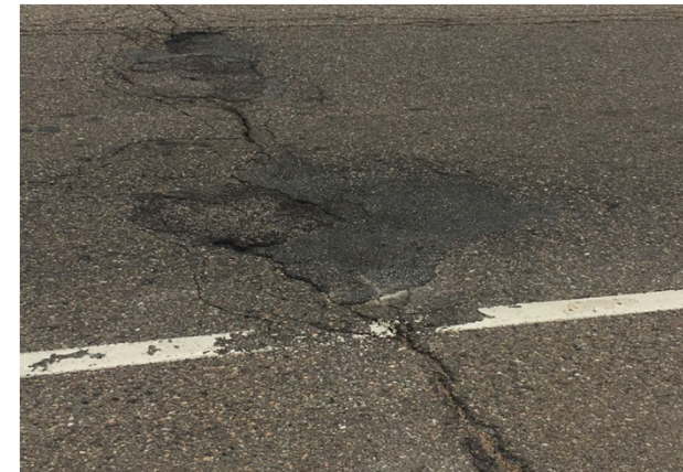
Poor pavement along a state highway
